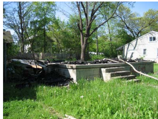
The foundation of 209 West Baker. Fire occurred here in a vacant and unsecured house on March 26, 2007. One firefighter suffered a burn during an offensive attack. At a subsequent fire on April 18, 2007, one firefighter suffered a shoulder injury during a defensive operation.
