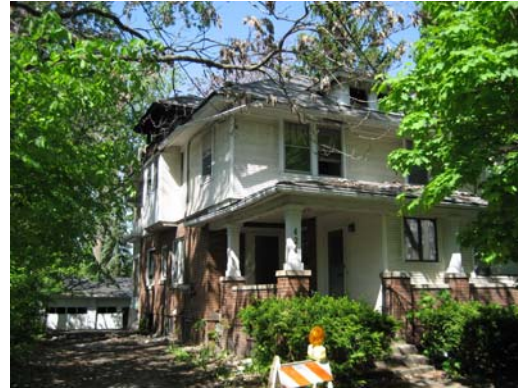
A vacant and unsecured house at 424 Thomson. Fire occurred here on March 4, 2007. One firefighter suffered a burn.
