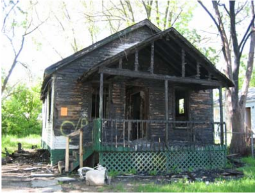
A vacant and unsecured house at 142 East Lorado. Fire occurred here on March 28, 2007. Defensive measures were initially used followed by interior overhaul. No firefighters were injured. The house is scheduled for emergency demolition.
